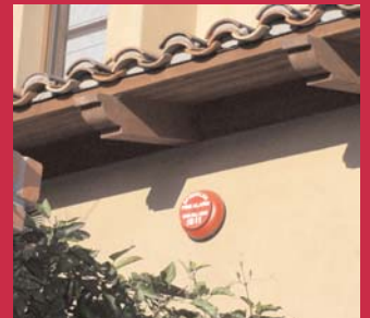
Residential fire sprinklers
